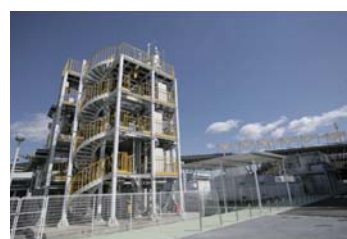
High-temperature gasification system
