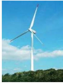
Alternative wind power generation, Used in Toyota Group Pavilion
