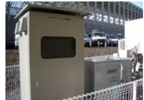
Fuel cell of Gas Pavilion
