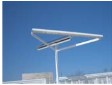
Solar cell panels on the roof
